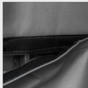
Heat insulation with durable fabric covering for improved service maintenance.
